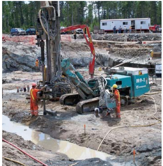
Drilling of piles at The Gathering Area — note bedrock outcropping in near background
