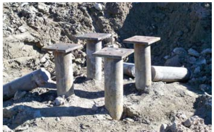
Piles cut down and awaiting welding of top plates at a typical PC-5 Pile Cap
