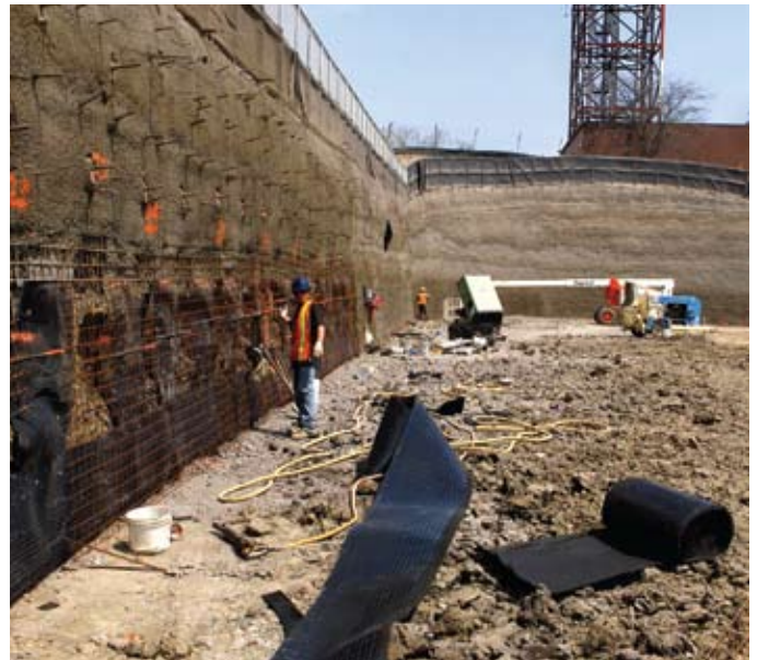
Third lift of eastern arm of wall excavated and ready for shotcrete installation
