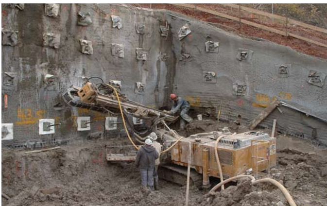
Versatile drill rig constructing soil anchors in tight quarters at southwest corner
