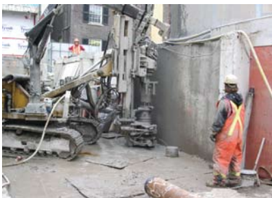
Construction of 273Ø micropile foundations for the new South Tower in open headroom within the former 1990's atrium footprint
