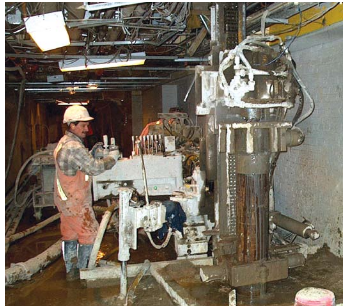
Construction of 273Ø micropile foundations for the new South Tower in low headroom inside the 1920's era ground floor space
