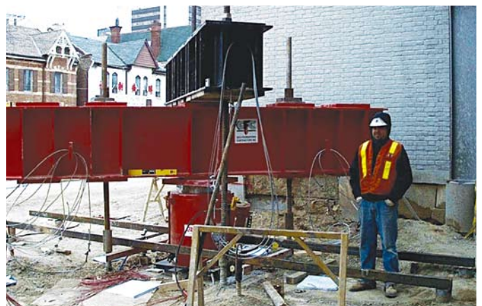
Static compression load testing to 8050 kN on a pile cap supported by a pair of 194Ø micropiles
