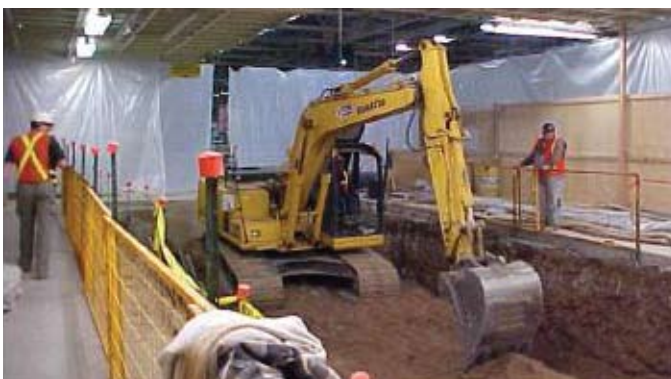
Start of pit excavating (by others) after installation of vertical soil dowels
