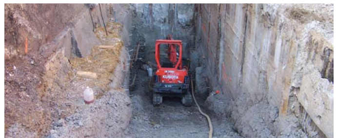
Drilling of fourth row soil anchors, using a customized, restricted access drill rig
