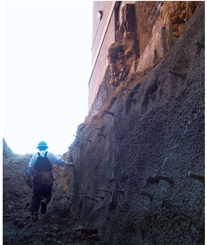
Anchored shotcrete wall system, underpinning heavily loaded spread footings, as seen from inside the 5m deep excavation
