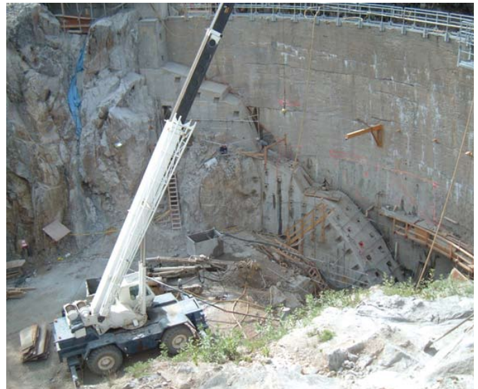
Downstream face of arch dam showing Plinths D (lowest) through A (upper left of photo)
