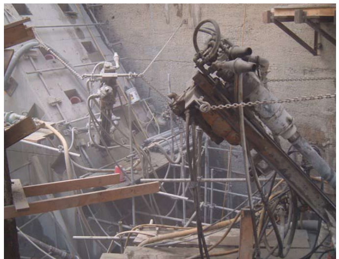
Two drills set up and drilling at Plinth E (right, foreground) and Plinth D (left, background)
