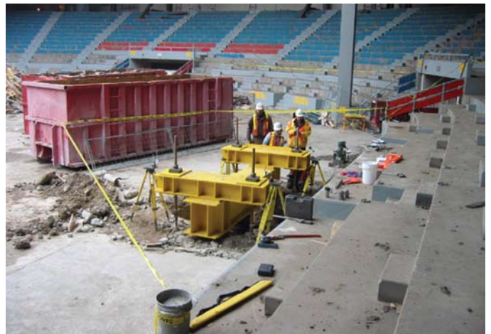
Static compressive load testing of a sacrificial micropile to 2590 kN (220% of design load)
