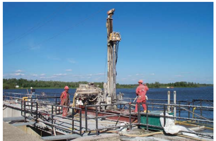
Rock anchor drilling in progress at log chute from atop temporary bridge
