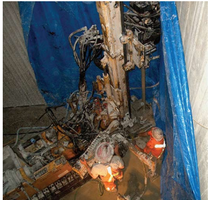
Installation of micropiles tight to the interior walls of the Science Centre
