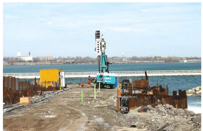
Drilling of 80-metre deep grout curtain holes from atop cofferdam rock fill
