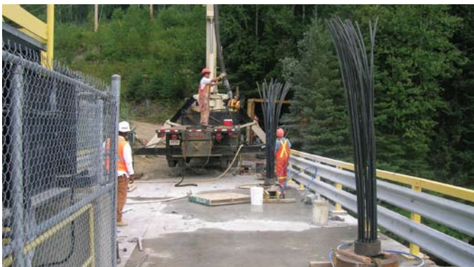
Installation by boom truck of Pier 3's 12-strand rock anchor – in foreground, Pier 1 (right) and Pier 2 rock anchors installed ready for grouting
