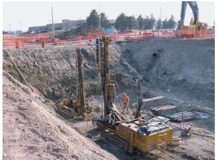
Compaction grouting pipes being installed by 2 drill rigs in the south-west quadrant of the intersection
