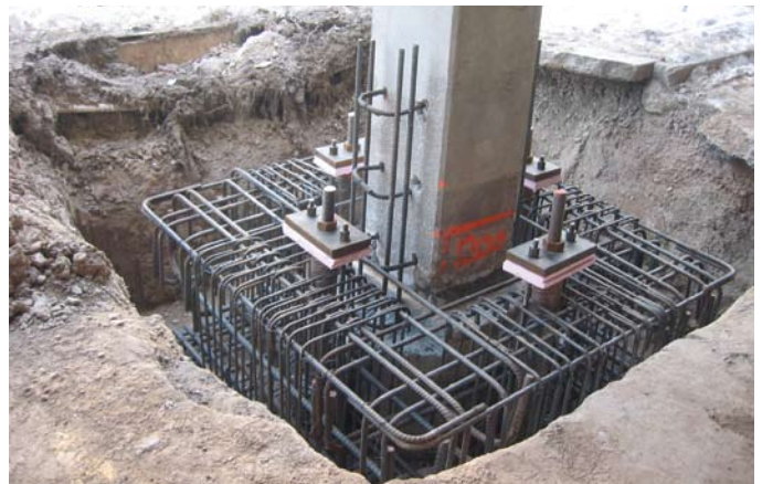
Pile cap reinforcement in place ready for concrete – each micropile is dressed with ducting and tension rods to enable pre-loading
