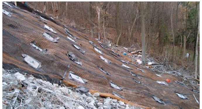
Slope face treatment – plates, geogrid, biomats - prior to final soil layer applications
