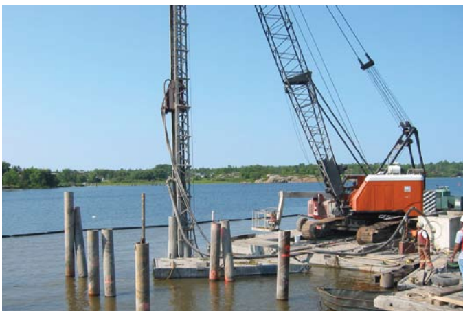
Pile installation in progress using swinging leads supported by a barge-based crane
