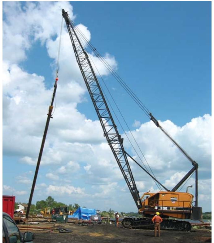
A 406Ø pipe pile, complete with drill rods and downhole hammer inside, being hoisted by land-based crane prior to positioning within barge-base swinging leads
