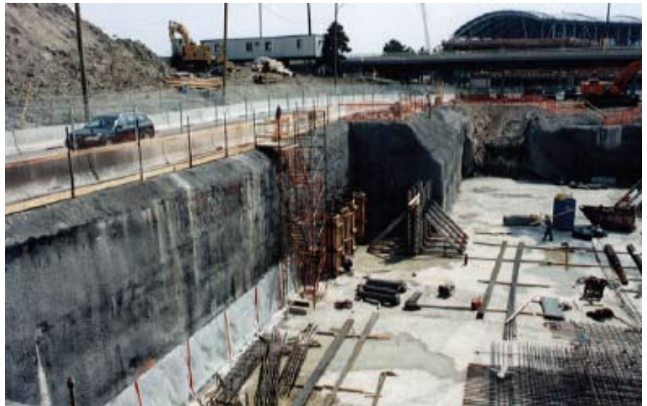
Excavation shoring complete – construction of reinforced concrete reservoir floor slab and walls in progress
