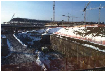
Anchored shotcrete shoring of 7m deep excavation with new mega-terminal construction in progress in background
